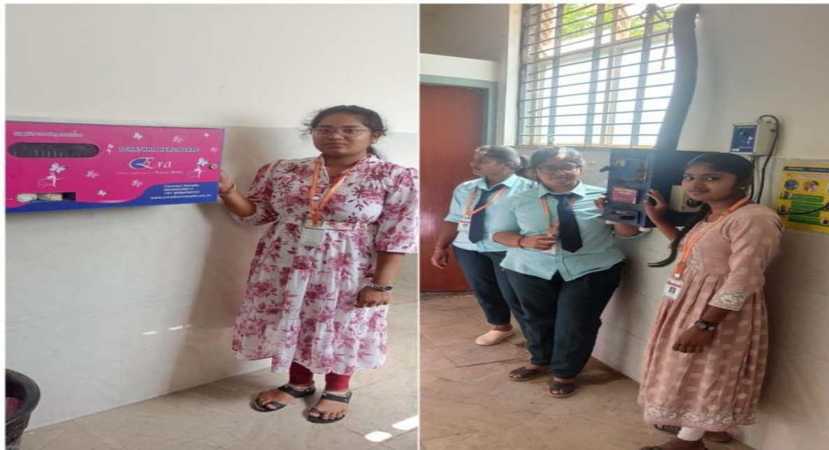
Sanitary Pad Vending Machine and Incinerator machine in the Ladies Wash Rooms
